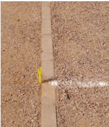
↑ Use of landscape blocks for shooting lines. PASEO VISTA RECREATION AREA , Chandler, Ariz.
