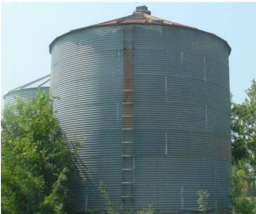
Enclosures with limited openings for entry and exit – such as tanks and silos – can hold many hidden hazards.
